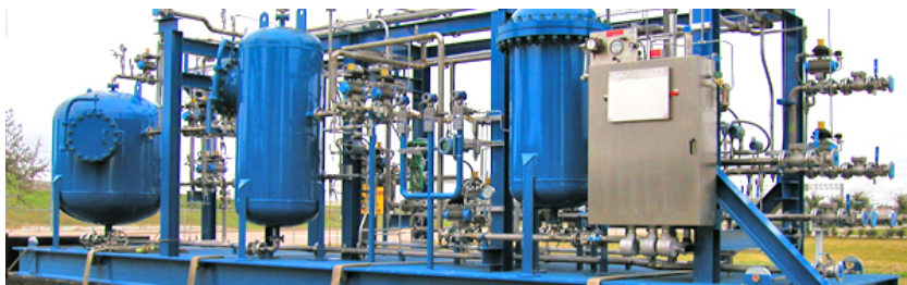
Elemental Sulfur Production in a Gas Treatment Plant
